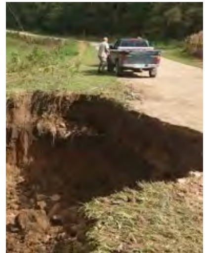
Flooding washed out road, Root River SWCD
